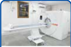
Rotary Rajkot Greater CT Scan Centre at B T Savani Kidney Hospital
